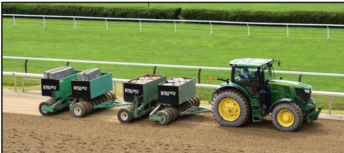
Figure 3. Rollers being pulled by a tractor over the Saratoga Main track to compact the freshly harrowed surface. (Photograph by Scott E. Palmer)
